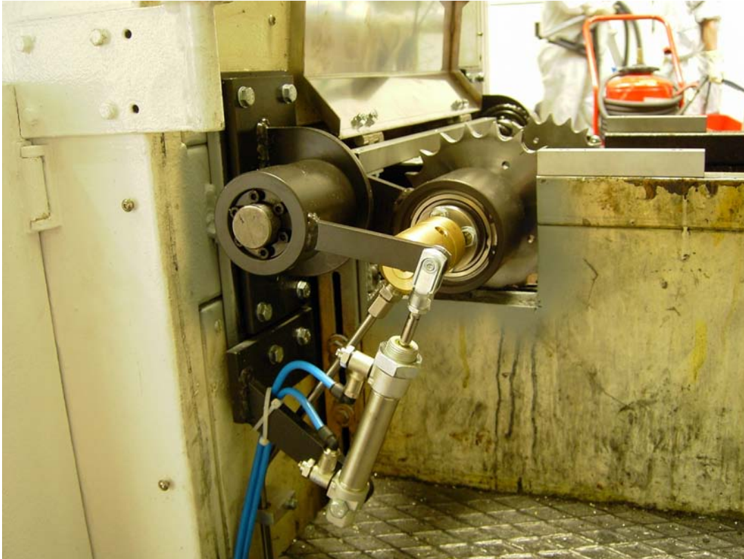
example of a drier, upgraded with a chain lubrication: bearing
